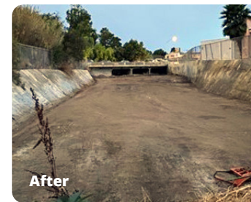
Channel Maintenance at Ocean View Channel to remove overgrown vegetation and debris to prevent flooding.
